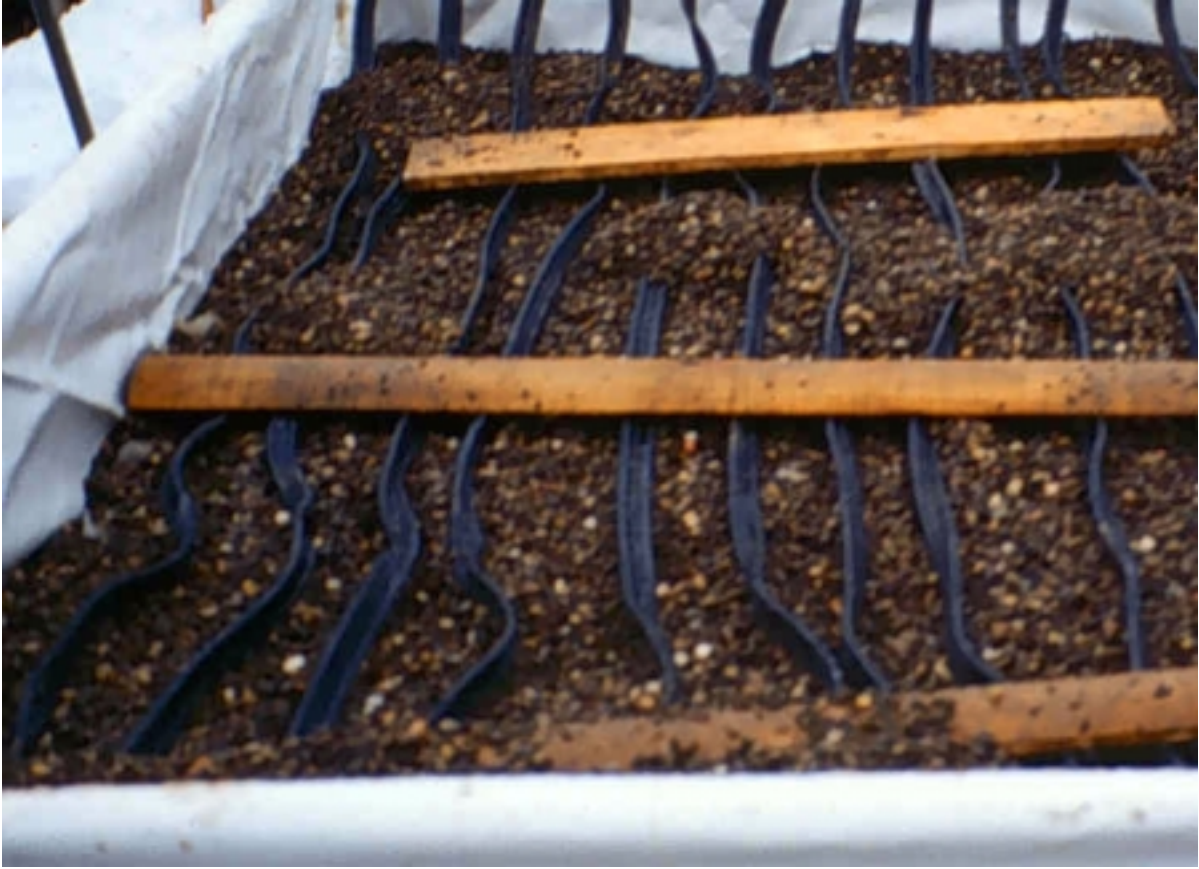
Picture 3 Illustration of the root-zone heating system buried in the gravel beds. Note boards were used to hold down the plastic tubing when filling the beds with gravel.
